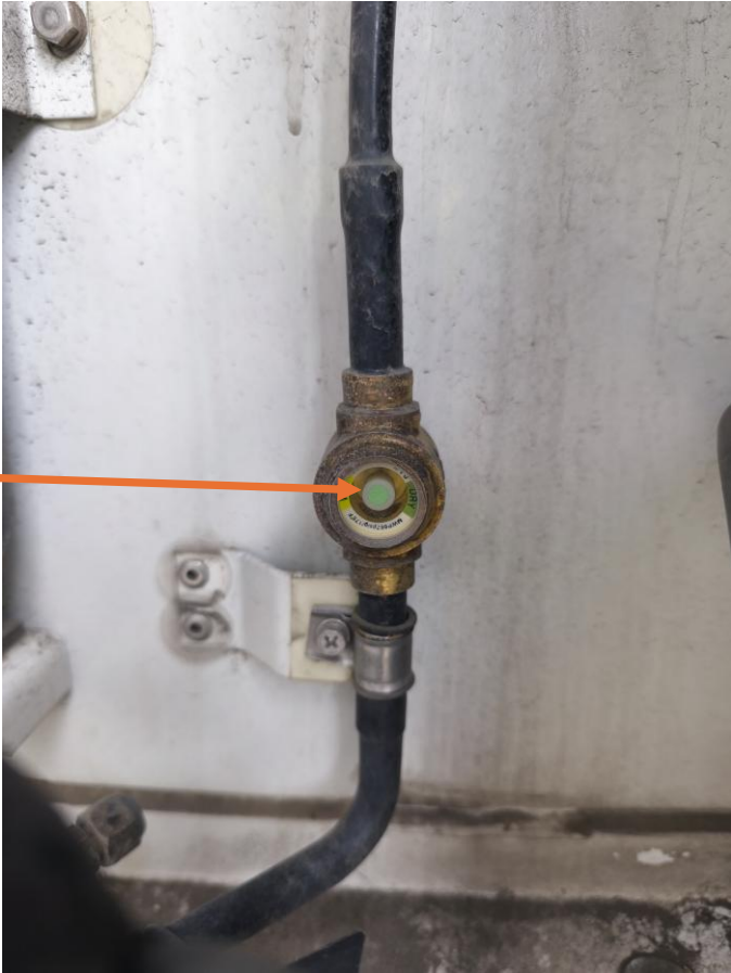
SGL Sight glass in Piping
