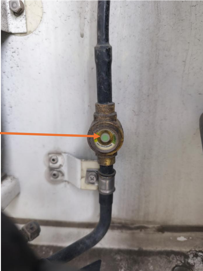
SGL Sight glass in Piping
